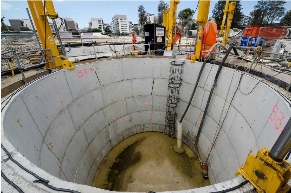
Caisson for Water Quality Improvement Device
